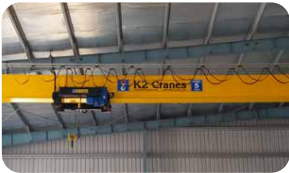
SINGLE GIRDER EOT CRANE
